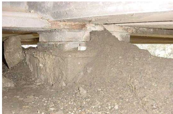
Figure 3.2.2 Debris and Sand Deposits around Bearing Seat Areas
